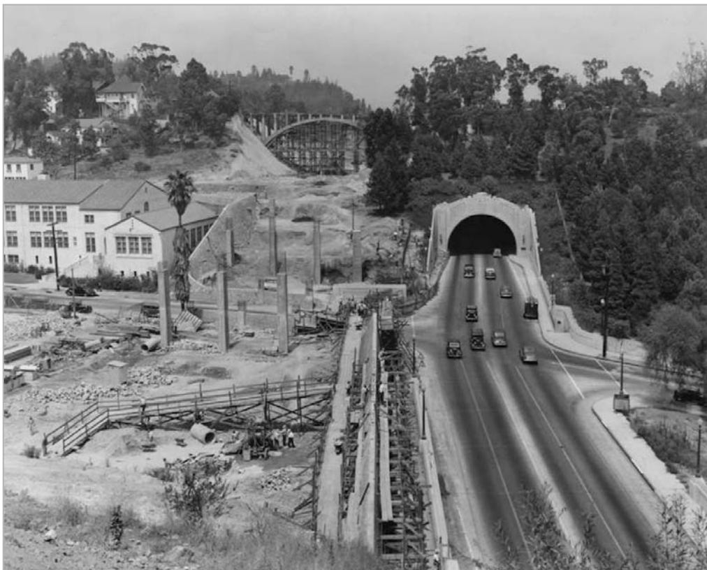
The Figueroa Street Tunnel during construction of the Arroyo Seco freeway through Elysian Park, circa 1941
