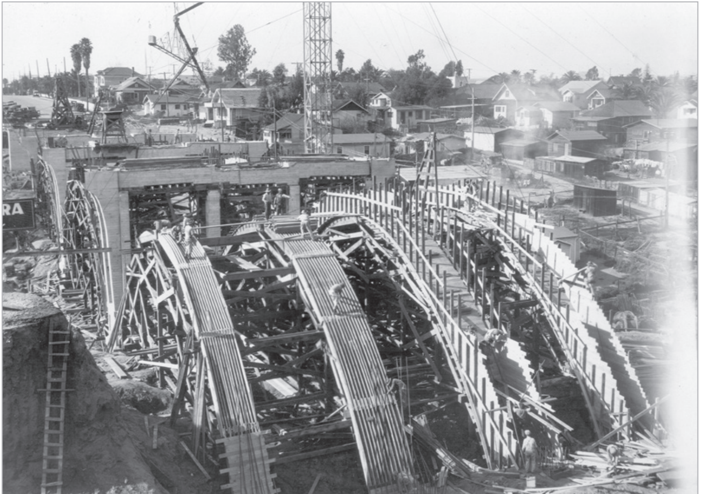
Lorena Street and Fourth Street bridge, closeup of arch rib from above, on the side of the street to the east (2/14/1928). (Photo courtesy Collection of Los Angeles City Archives Department of Engineering Historical Photos)
